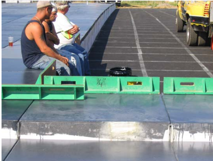
(b) EMAS Installation Processes at the Roanoke Regional Airport Courtesy of Alex Plaza
