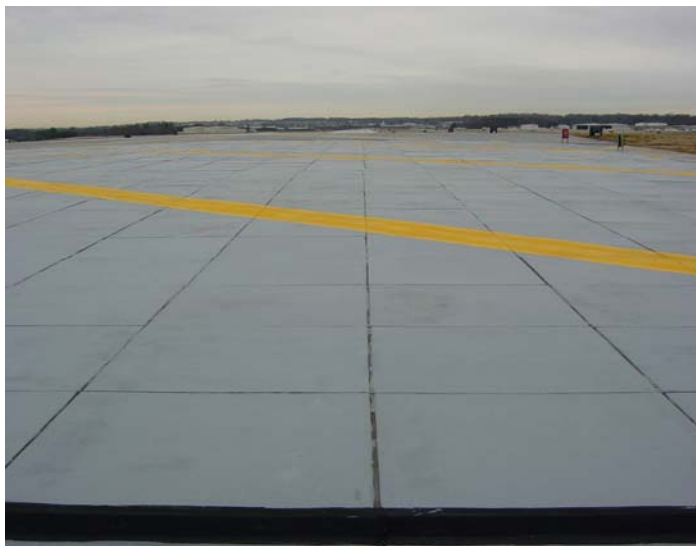
(c) EMAS Installed
